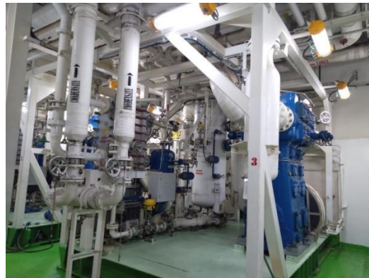
Gambar 5. Reliquefaction Plant LPG/C Gas Walio
